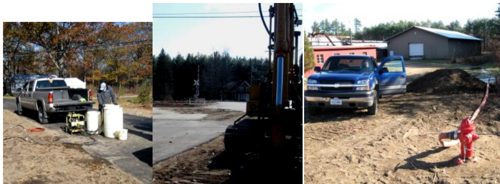
L to R— Disinfecting; water line crossing at RR crossing; testing water on south side of Rt. 2
